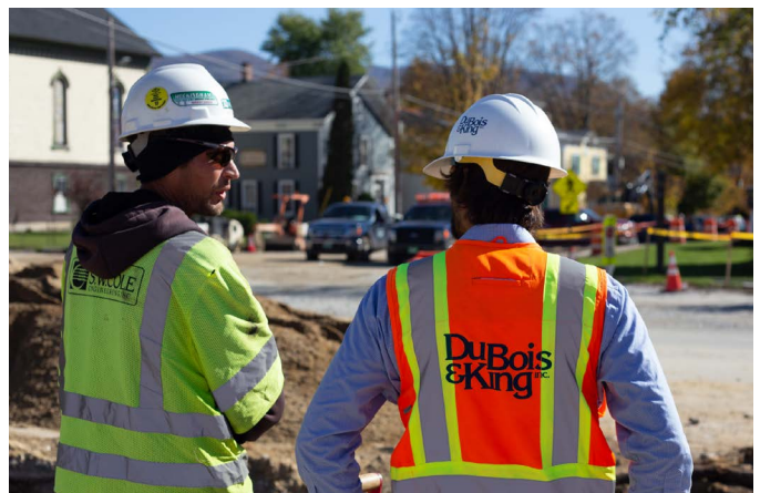
S. W. Cole and D&K worked closely together on the recent $20M US Route 7 Segment 6 project in downtown Brandon.
